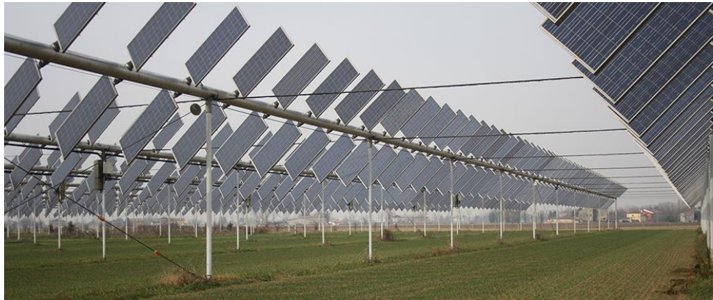
Figure 3: Technology 1.0 installed in Viriglio (Mantova, Italy)
