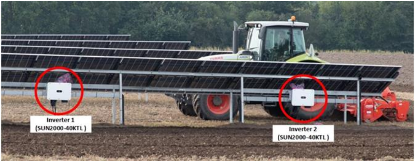
Figure 30: Inverters in field.
